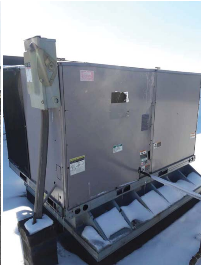
RTU above/serving the laundromat below
