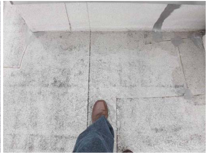
Standing water present outside the elevator shaft
