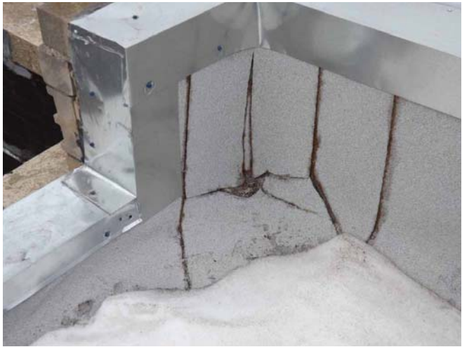
Amateur/improper wall flashing detail at inside corner
