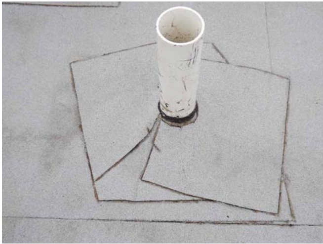
Amateur/improper flashing detail at 'P' vent
